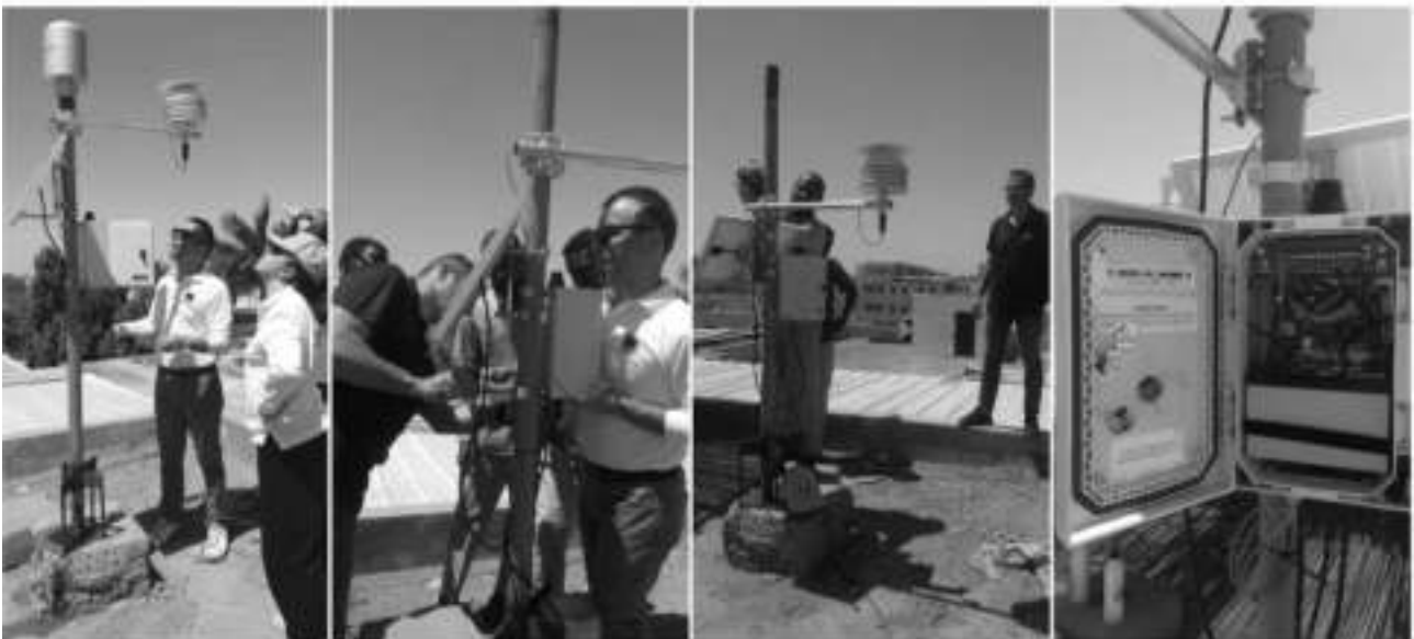
Figure 12: Installation of the weather station on the roof of AICS office in Khartoum.
